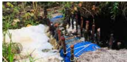
Figure 3-24: Sandbag block wrapped in tarpaulin sheet to prevent erosion when water flows over it
