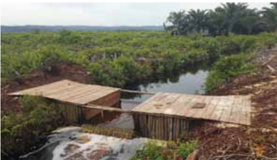
Figure 3-26: Center overflow in timber box block to allow small boat to pass through (Source: Ministry of Environment and Forestry, Indonesia) (Note: Low level of this spillway means the upstream peat is not fully rewetted).
