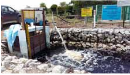
Figure 3-22: Gabion and watergate with water being supplemented by adjacent tube well (Note: Gabion structure, with large rocks, is not appropriate as it lets water pass through the rocks and bypass the gate)
