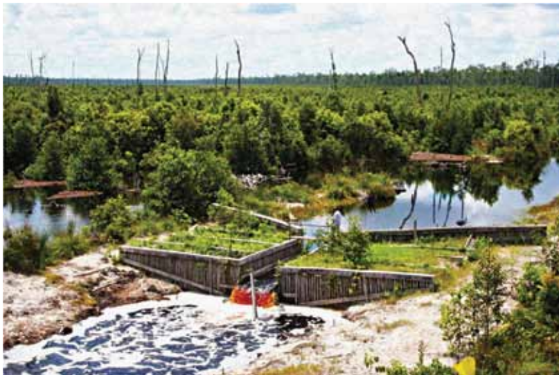
Figure 3-10: Dam constructed to block a former logging canal to restore peat swamp water levels.
