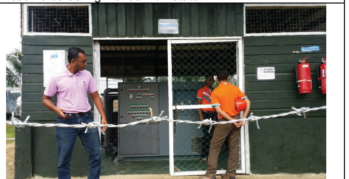
Water treatment plant using membrane technology for domestic water supply at Morisem 2 Estate.
