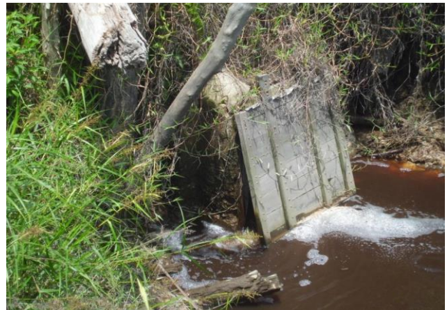
The Flap Gates open automatically during low tide, allowing drainage.
