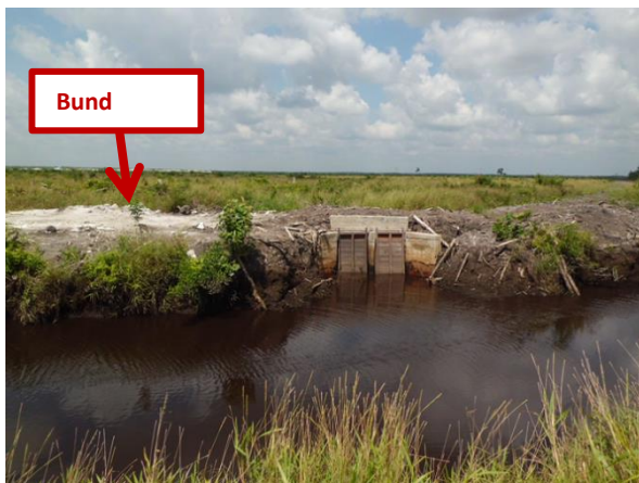
System with Bund and Flap Gates. The Flap Gates open automatically during high tide, preventing influx of tidal water.
