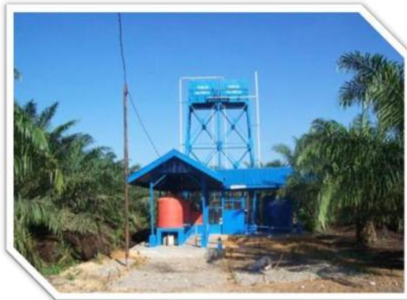
Water Filtration Plant
