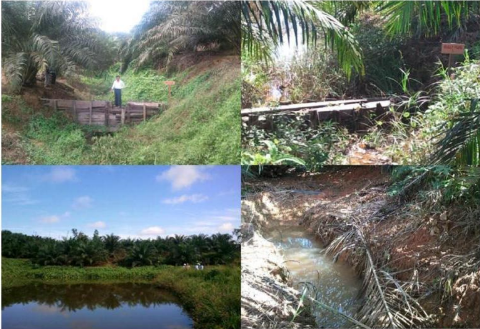
The civil engineering structures are functioning properly to achieve their purposes: the Retaining Dam (above-left), the Gully Plug (above-right), the Water Reservoir
