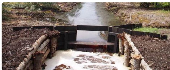
Figure 3-5: More sophisticated (but still low cost) structures on collection drains can be constructed with earth fill and wooden boards (example from United Plantations, Malaysia).
