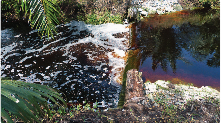
Figure 7-4: One weir installed at every 20 cm drop in water level to enable water retention along collection drains.
