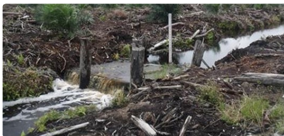
Figure 3-4: Water control structures do not need to be expensive structures and can be simply constructed with wood or sand bags.
