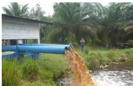
Figure 3-10: Pumping water to a canal to raise water level in particular during dry season.
