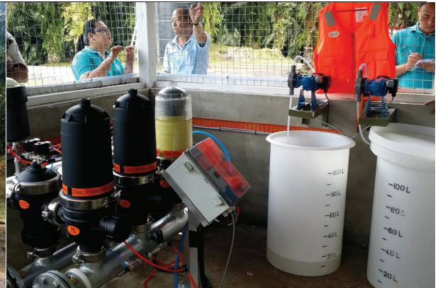
New Water Treatment plant installed near linesites at Syarimo estates.
