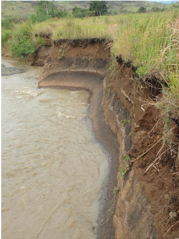
Figure 9 River bank erosion on Beboi Creek, the IMPU is on the RHS.
