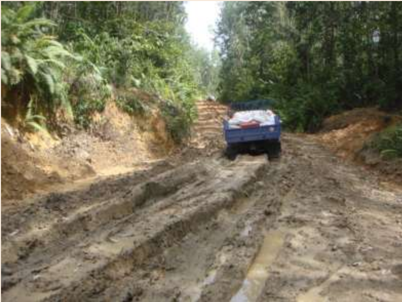
Poor condition of old timber road from Rh Iba to Keresia Plantations
